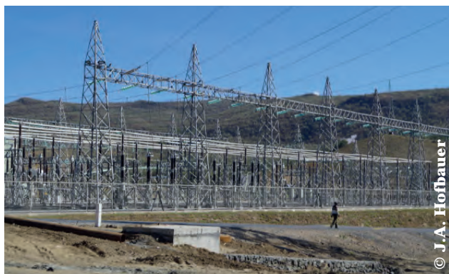
Olkaria geothermal plant, Kenya.
